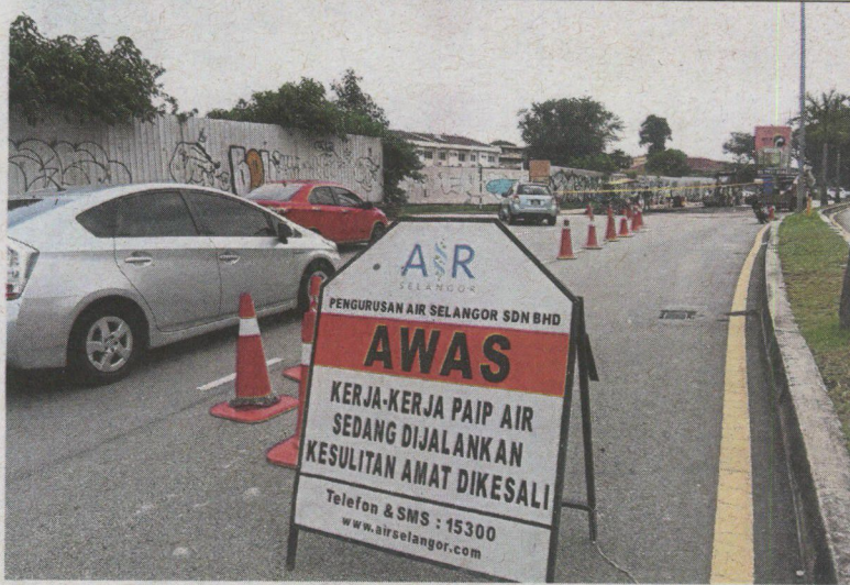
Part of Jalan Universiti, Petaling Jaya was closed to motorists following a burst pipe incident on Wednesday.
