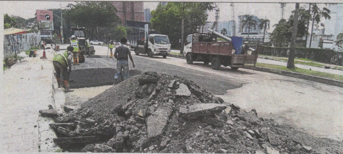
Air Selangor contractors resurfacing the affected area along Jalan Universiti in Petaling Jaya after completing repair works on the pipe yesterday.
